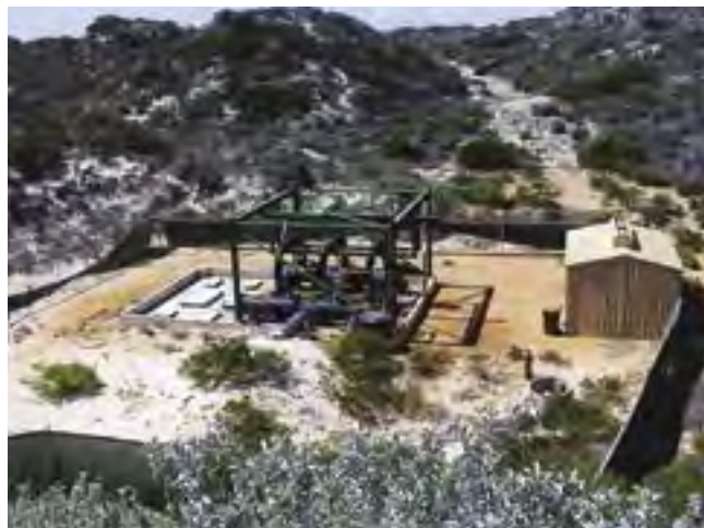
Figure 17. Cognis Pty Ltd, pumping station.
